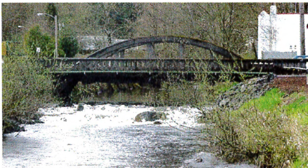
As the gravity flow pipe was exposed, the cascade just downstream of the bridge enlarged.
