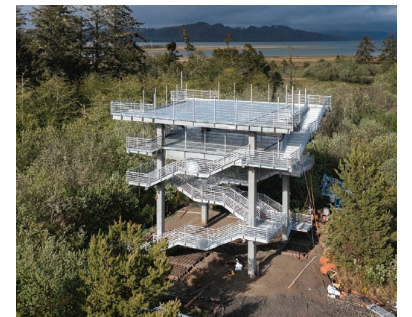
In 2021, the Shoalwater Bay Tribe partnered with Washington’s Emergency Management Division and FEMA to construct a tsunami evacuation tower to keep the community safe in the event of earthquake and tsunami.
